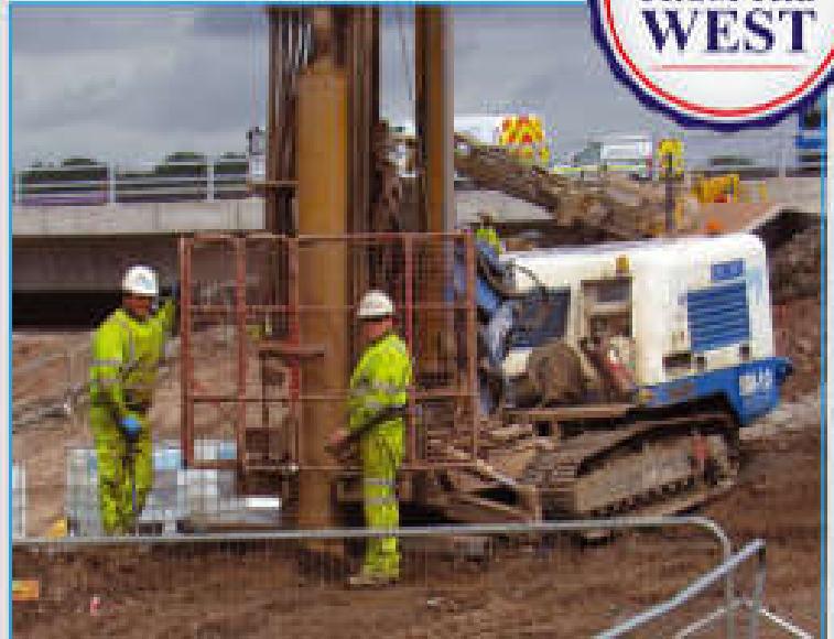
Martin Barton (Drilling Assistant) (left) and Danny Ashton (Lead Driller) enjoy a rare moment of sunshine during the installation of a dewatering well for the underpass.
